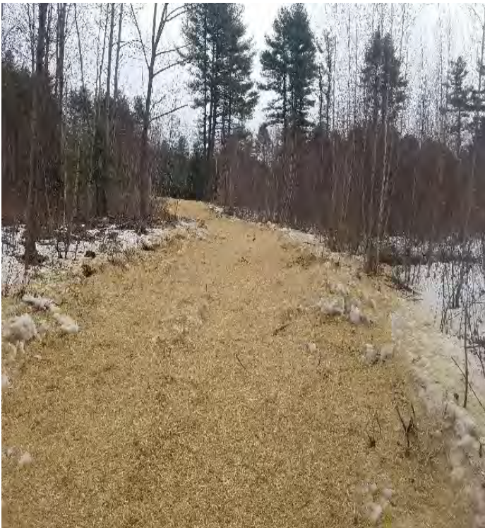
Fig 23: Straw spread over access road leading to Str. 10, off of Route 4. Viewing east. (01-14-20).
