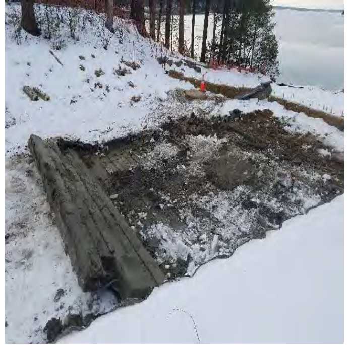
Fig 2: Removing timber mats from Gundalow landing/east side of the Bay. Viewing south. (01-10-20).
