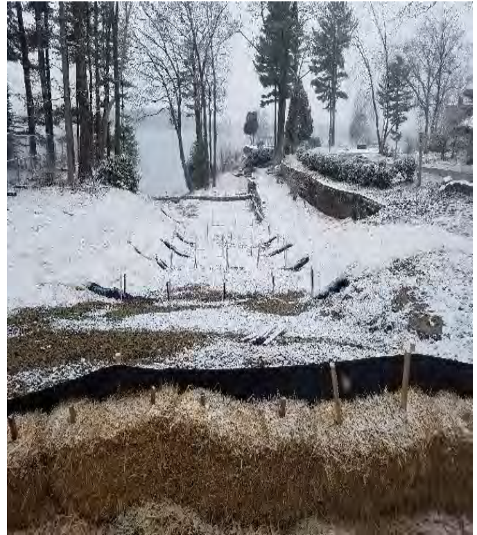
Fig 14: Finished winter stabilization and required BMPs at Gundalow Landing/east side of the Bay. Viewing west. (01-13-20).
