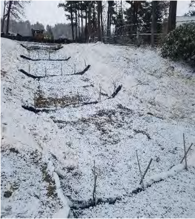
Fig 13: Finished winter stabilization and required BMPs at Gundalow landing/ east side of the Bay. Viewing east. (01-13-20).
