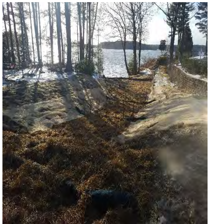
Fig 12: Crew installing BMPs on slope to vault at Gundalow landing/ east side of the Bay. Prepping for weekend rain. Viewing west. (01-11-20).
