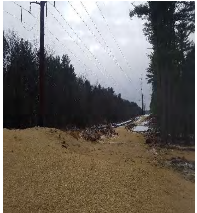
Fig 24: Strs 11 and 12. Viewing south. (01-14-20).
