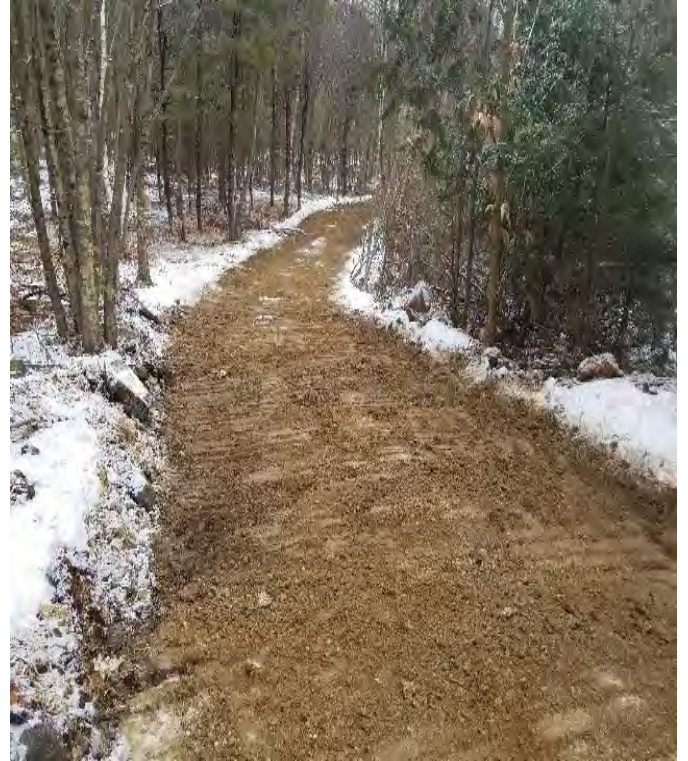
Fig 22: Removing mats on access road leading to Str. 10, of off route 4. Viewing east. (01-14-20).
