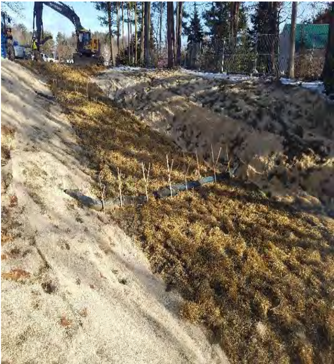
Fig 11: Crew installing BMPs on slope to vault at Gundalow landing/ east side of the Bay. Prepping for weekend rain. Viewing east. (01-11-20).
