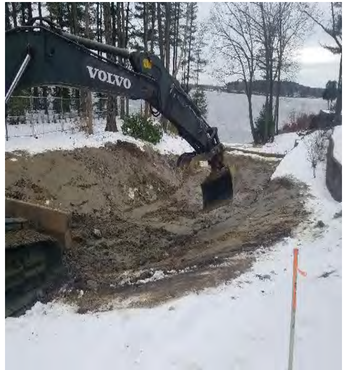
Fig 4: Restoring and shaping slope and banks at Gundalow landing/east side of the Bay. Viewing west. (01-10-20).
